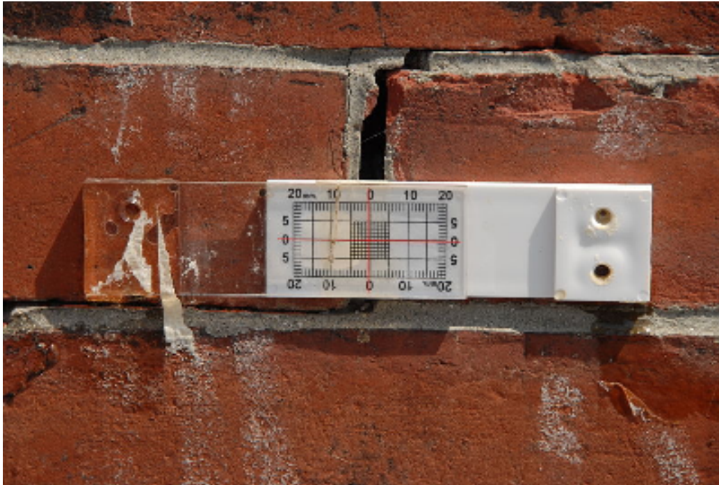
Mechanical strain gauge used to measure the growth of a crack in a masonry foundation. This one is installed on the Hudson-Athens Lighthouse. Photo by Roy Smith, used with permission.
