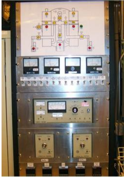
Wired relay type panel
