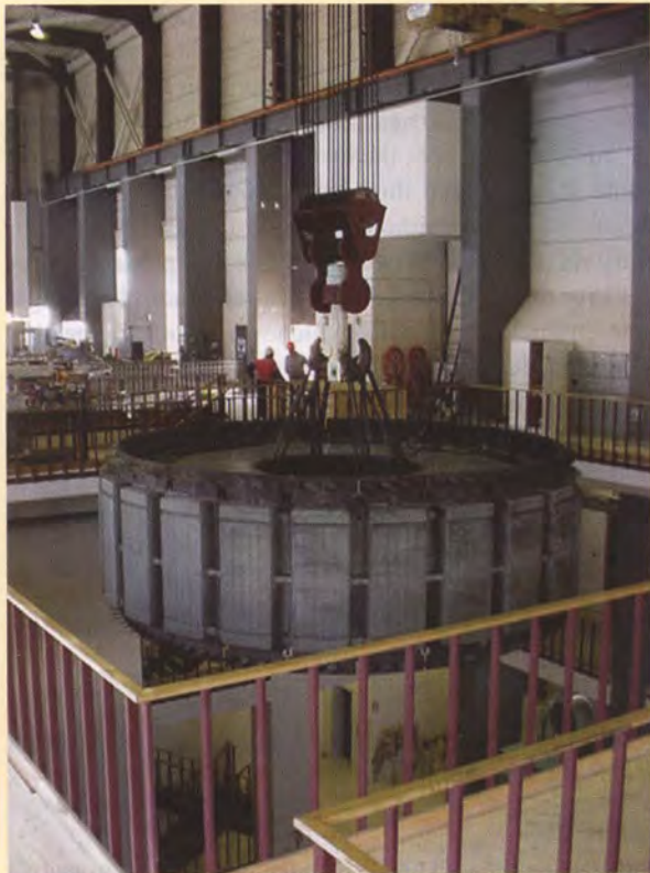
FIGURE 12.21 The 24-pole rotor of a synchronous generator as it is being lowered into position. Photo courtesy Dr. Wade Enright, Te Kura Pukaha Vira O Te Whare Wananga O Waitaha, Aotearoa.
