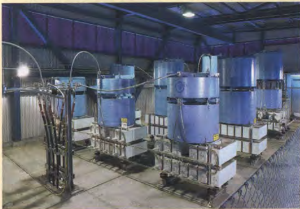
■ FIGURE 11.20 A compensation capacitor installation. (Courtesy of Nokian Capacitors Ltd.)
