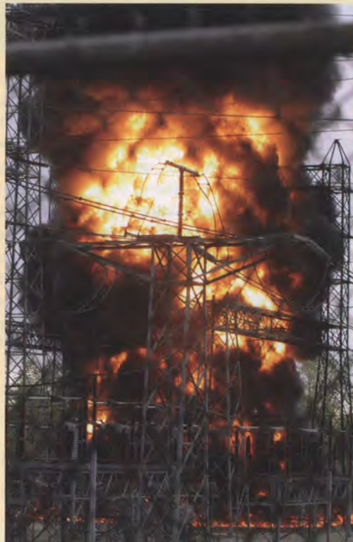
■ FIGURE 13.28 Fire that broke out in 2004 at the 340,000 V American Electric Power Substation near Mishawaka, Indiana. © AP/Wide World Photos
