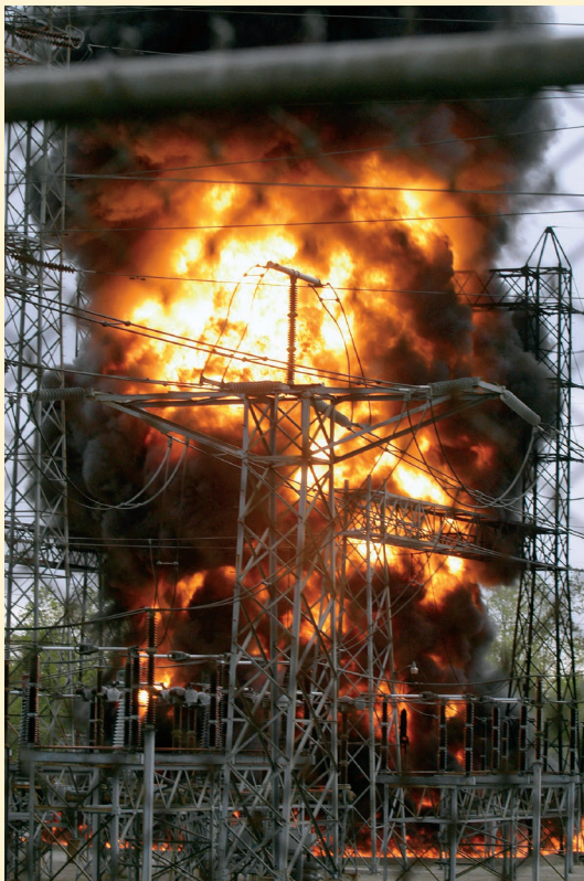
■ FIGURE 13.28 Fire that broke out in 2004 at the 340,000 V American Electric Power Substation near Mishawaka, Indiana. (©Greg Swiercz/South Bend Tribune/AP Images)
