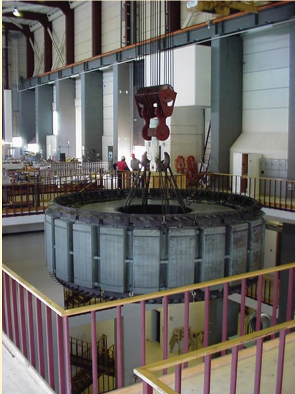
■ FIGURE 12.21 The 24-pole rotor of a synchronous generator as it is being lowered into position. (Courtesy of Dr. Wade Enright, Te Kura Pukaha Vira O Te Whare Wananga O Waitaha, Aotearoa)
