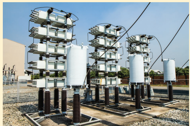
FIGURE 11.21 A compensation capacitor installation. (©Kitja Chavanavech/123RF)
